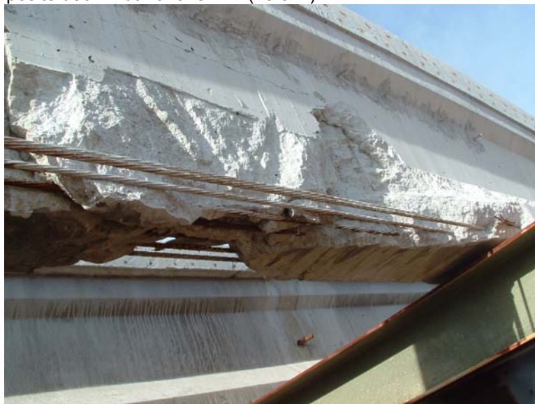
Fig. 1 AASHTO1 at NCDOT yard after impact damage.
