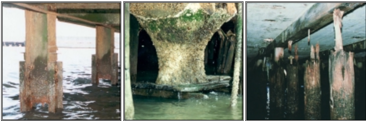
a) Corroded steel piles b) Degraded concrete pile c) Deteriorated timber piles
